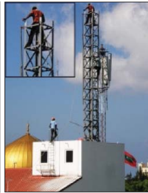
Technicians with no safety equipment or measures - a common sight in Maldives
