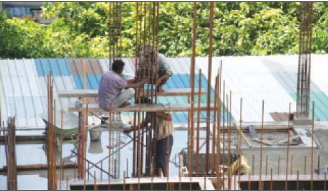
Construction workers working with no safety equipment or measures
