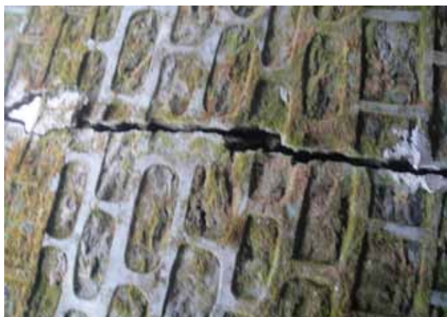
A cracked wall seen at the prison during the monitoring by the NHRC team, Khotang Office
